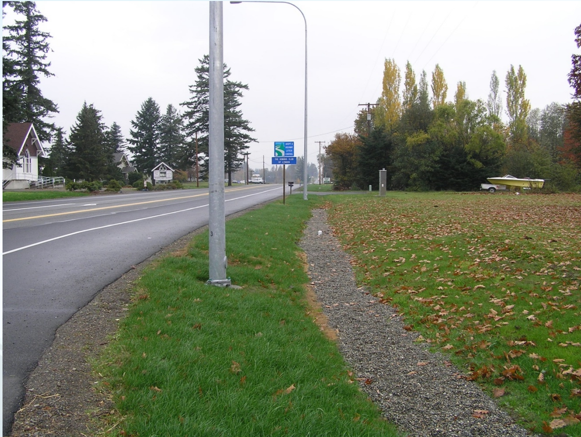
Infiltration Trench with Filter Strip (SR 539)
